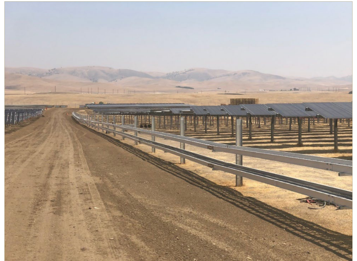
Photo credit: First Solar. Wiring is installed in above-ground trays instead of below-ground trenches
